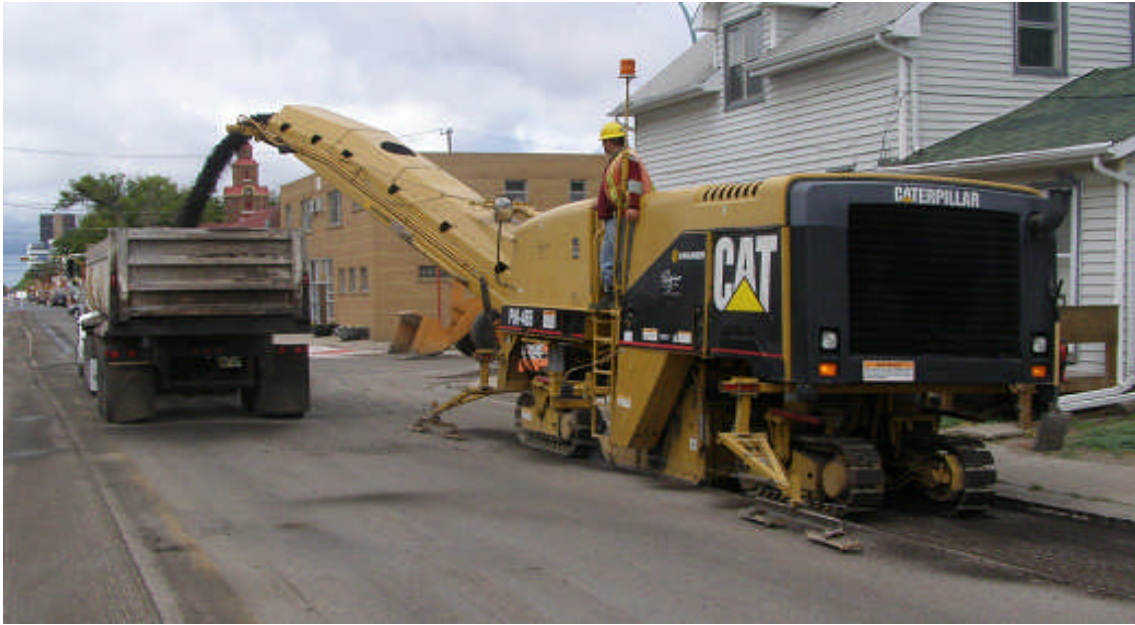
The asphalt paver crew performing precision asphalt cutting - preparing the road surface for repaving.
