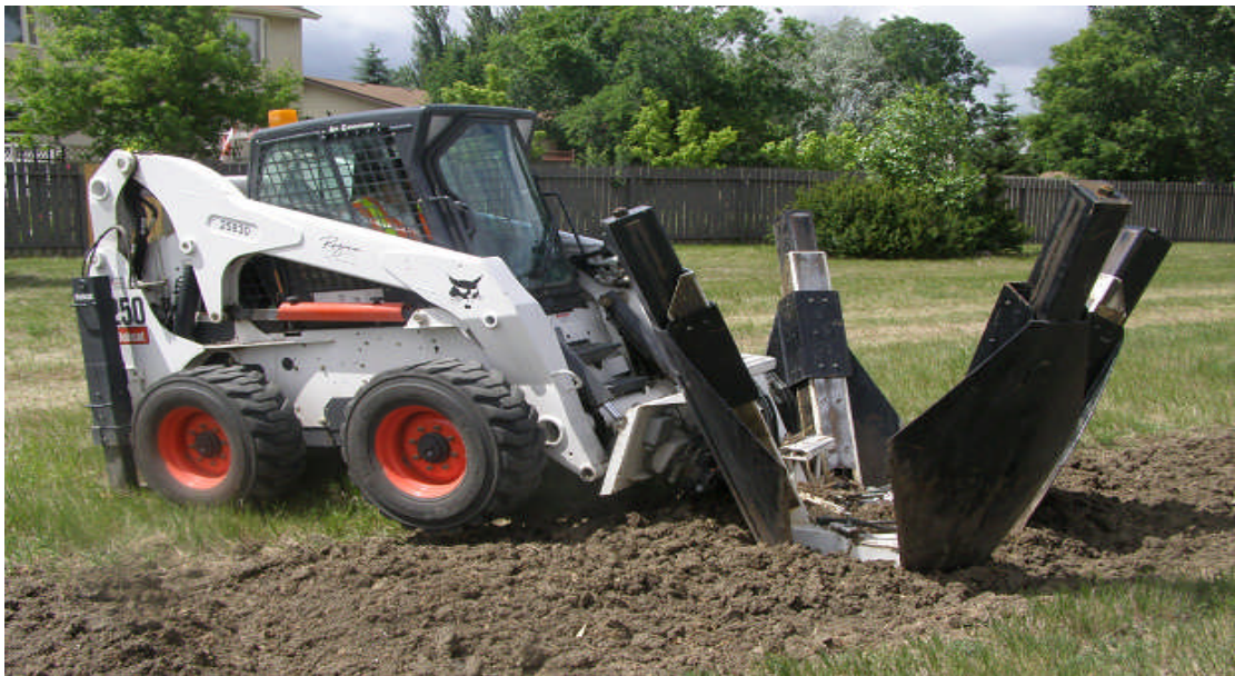
Tree spade unit - excavating a deep enough hole to plant trees in the SE section of the city.
